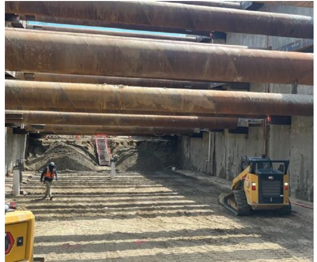
Fine grading excavation in preparation for ramp slab to be poured in this section
