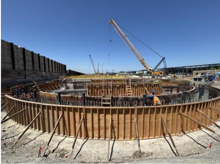
Rebar and formwork installation on top portion of caterpillar portion of the launch structure
