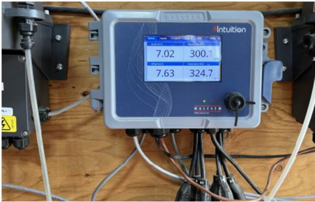
pH Level and Flowrate Readings at Influent Groundwater Treatment Plant
