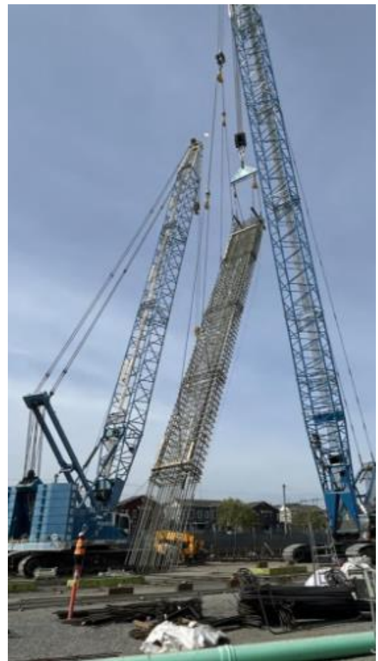
Lifting Upper Section (Glass Fiber Reinforced Polymer Section) of Rebar Cage for Cat Shaft D-Wall Panel
